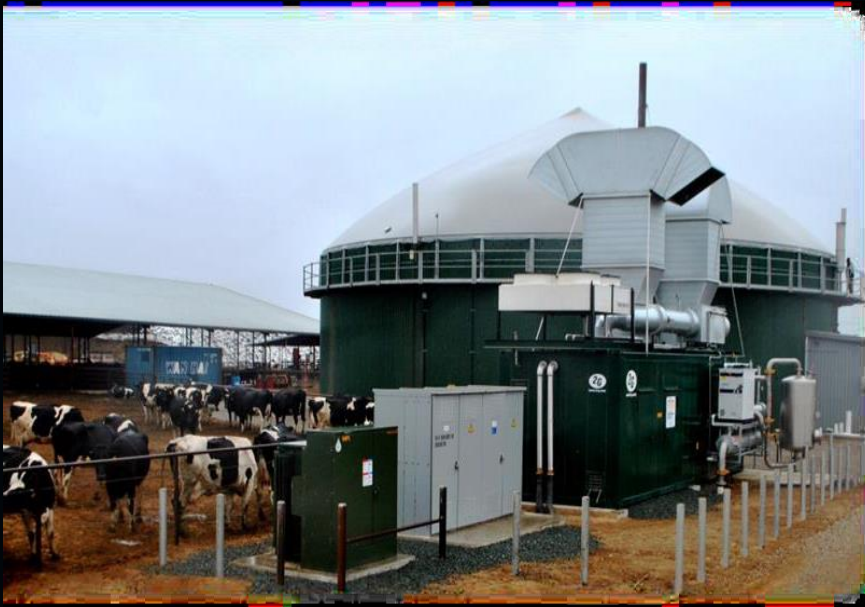
biogas digester at New Hope Dairy in Galt, Calif http://cdrf.org/wp-content/uploads/2014/12/DairyCares-MOR-11-14.bmp
